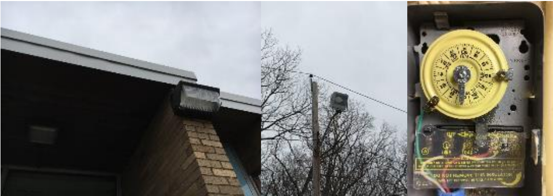
Figure 11-Exterior Lighting and Timeclock Control
