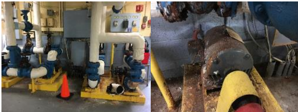
Figure 13-Hot Water Pumps and Motors
