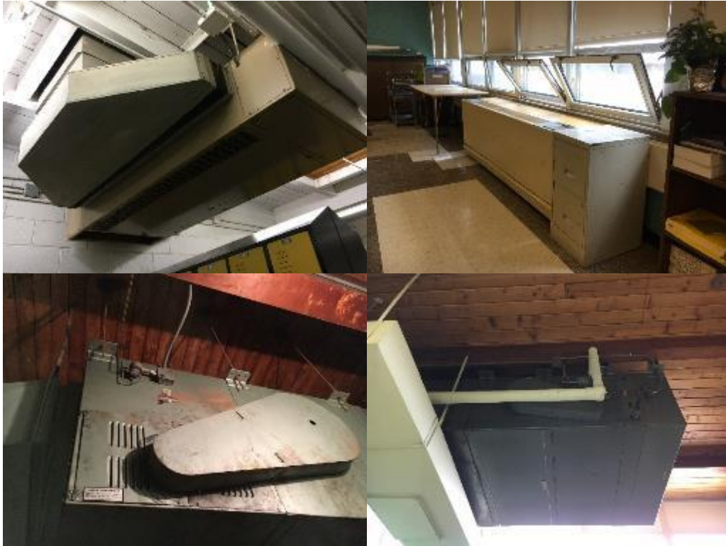
Figure 14-Unit Ventilators and larger Heating-Ventilation Units
